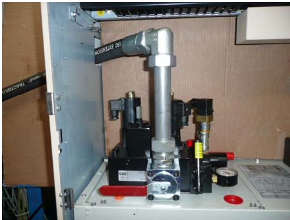
Typical MRC installation without DLV A3 safety valve fitted.
